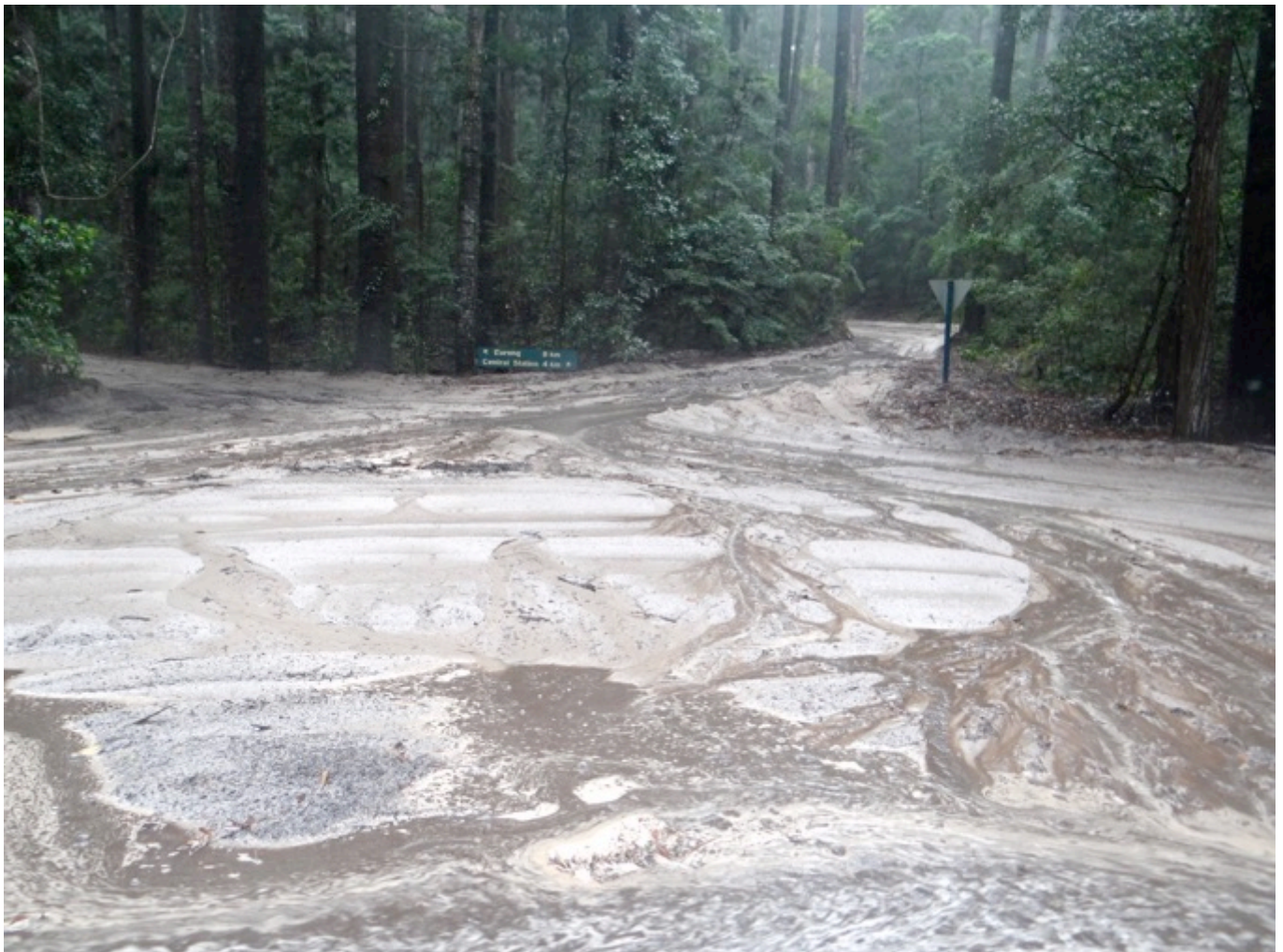
Sediment movement observed at the intersection of Central Station Eurong and the link road to Lake McKenzie
