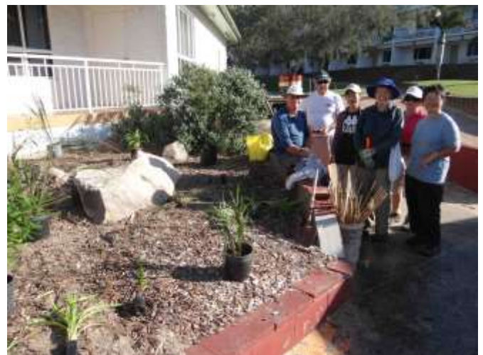
The team about to plant the front garden at the entrance of Eurong Resort with island grown plants supplied by Kingfisher Nursery
