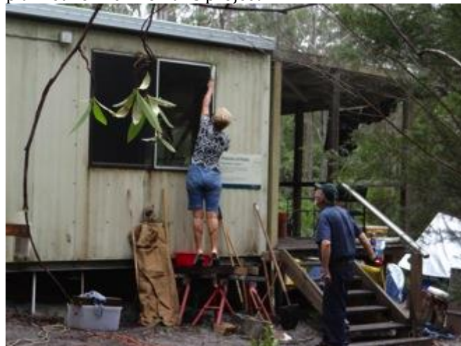
Jennifer McDonald's cleans a window beside a Friends of Parks sign. Harold Charles who has overseen all of the building renovation work is just checking.
