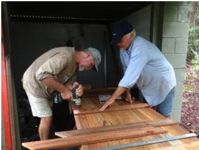
Noel and Eric using up the last of the power to complete the doors to secure the Generator shed
