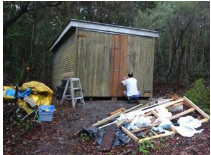
Neville works on the doors of the storage shed that was almost overgrown before our arrival
